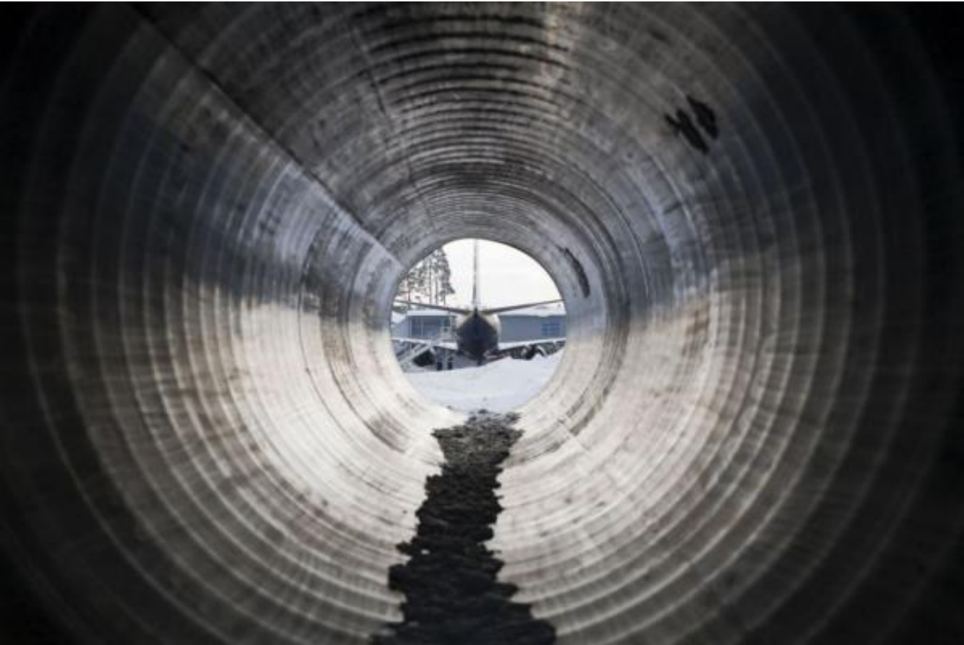
Uponor soil drainage system big profile pipes in Skavsta Airport, Nyköping
