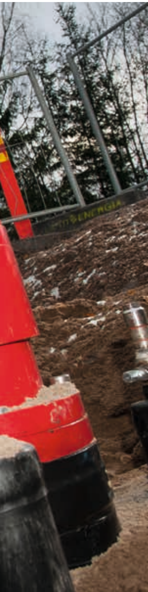
Lahti Energia's Kaj Åberg and KWH Pipe's Jan-Erik Svarvén point out that remote control makes operation easy and trouble-free.
