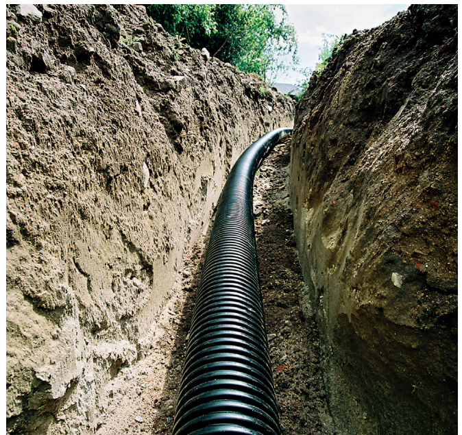
Even the installation of large pipe lengths of up to 200 m is child's play with the Ecoflex decoiler.
