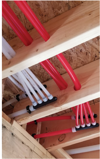
Figure 6-7: Bundled Uponor AquaPEX Pipe
