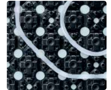
Uponor PE-Xa pipe installed at 45° angles
