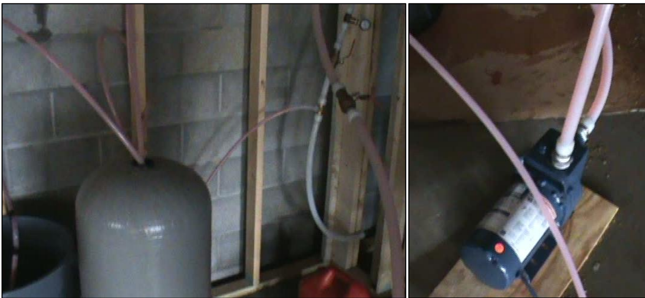
Figure 1: Storage Tank and Jet Pump
