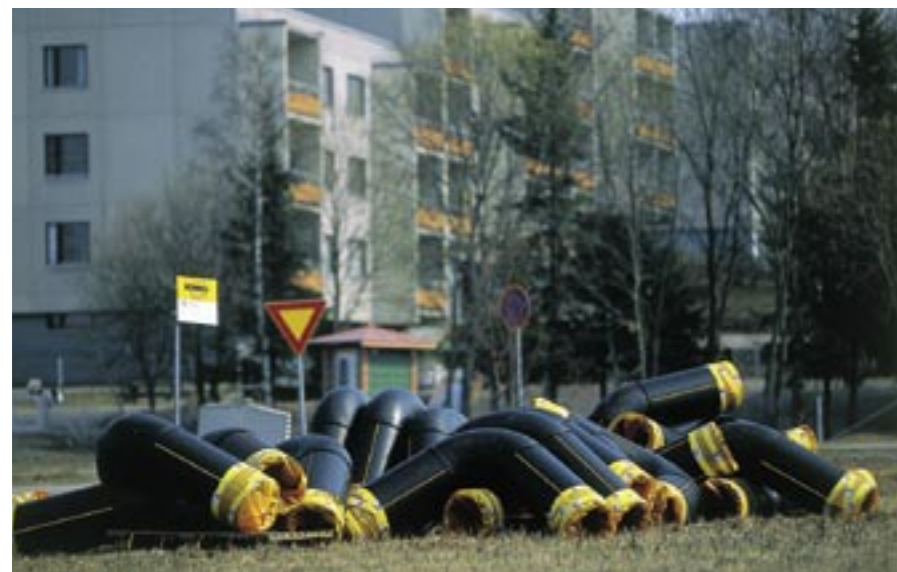
The gas pipe was laid in Espoo during the spring at a brisk rate of 400-600 metres per day.
