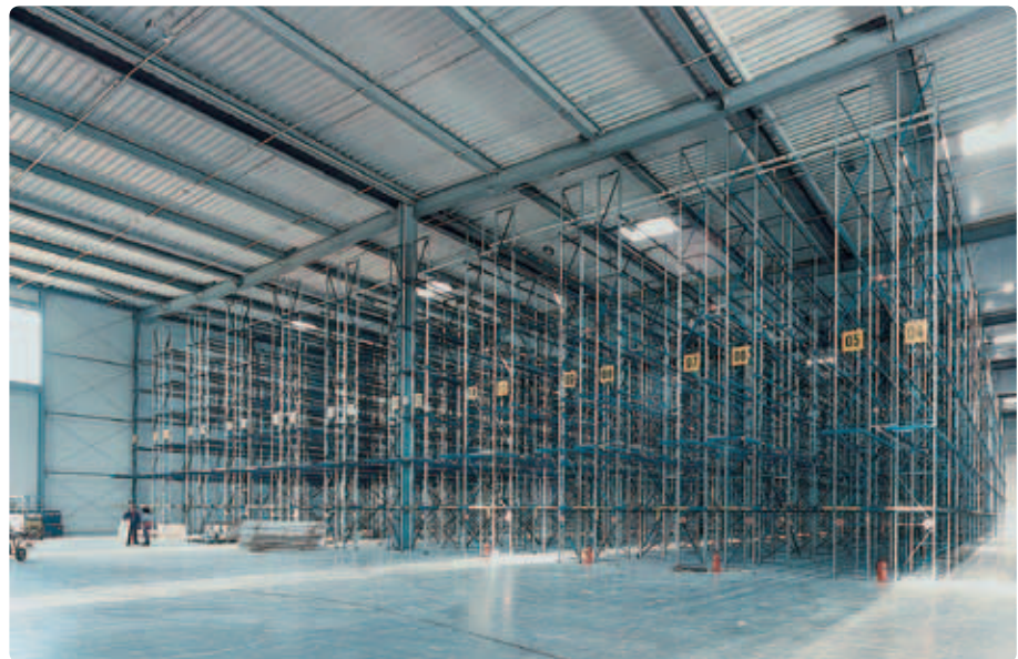
20,000 m 2 Uponor industrial underfloor heating in a high rack warehouse in Hückelhoven, Germany
