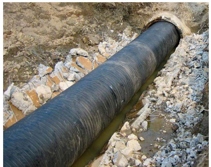
Hämeenlinna, Finland: A highway crossing was renovated by sliplining a Weholite pipe DN/ID 1000/1125mm into a concrete pipe DN 1300mm. Jointing type: Extrusion welding. Total length 750m.
