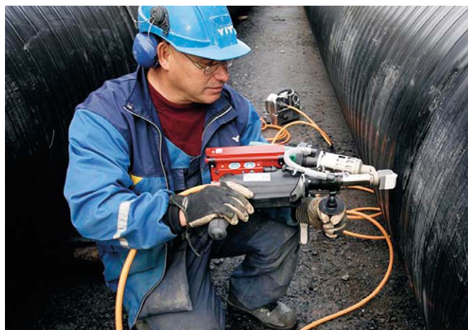
Hand-held extrusion machine. Hand extrusion is especially suited for waterproofing thread joints.
