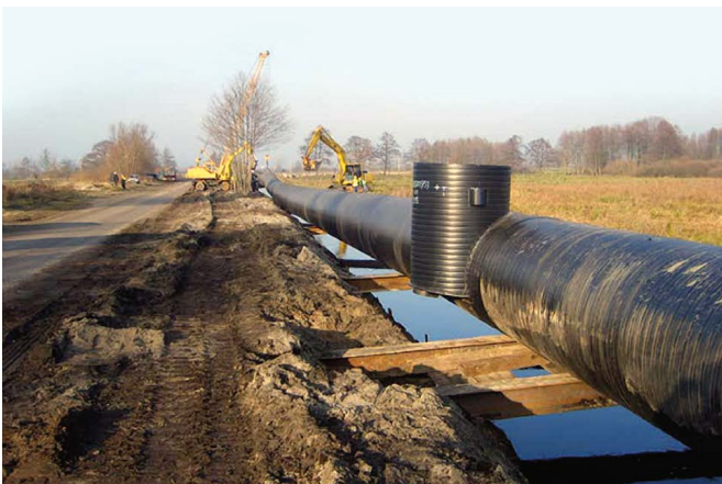
Gdynia, Poland: Wastewater treatment plant discharge pipes. Uponor delivered 2257m Weholite pipes DN/ID 1400–1500mm and 22 manholes. To facilitate installation, most pipes were delivered in 15m lengths.
