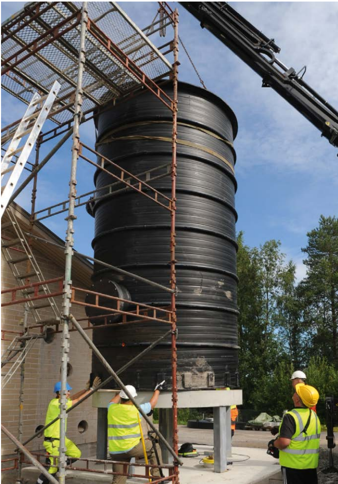
Iisalmi, Finland: An insulated aeration tank removes excess carbon dioxide from the water. The prefabricated DN/ID 2400mm tank was installed above-ground on a concrete slab.
