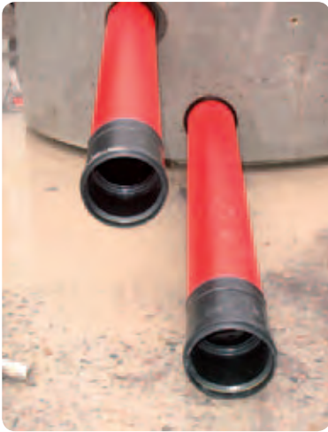
Figure 8.2.14. Tripla lead-through into a concrete chamber.
