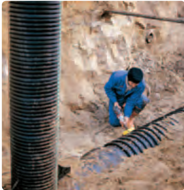
7. After final backfill and compaction, the pipe interior is inspected as necessary, for any deformation and for angular deflection of the joints.
