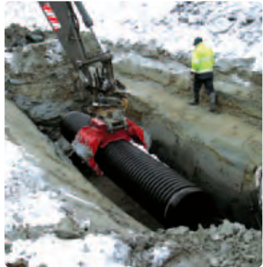
In the case of deeper trenches, a pipe grapple can be used as an excavator attachment for safer pipe placement.
