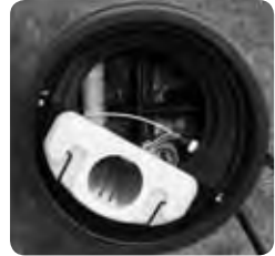
The chemical is dosed in the first tank chamber.
