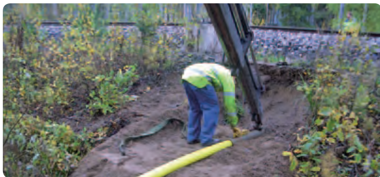
Figure 8.2.25. Preparing to mole Tripla pipe beneath a rail line. Moling distance 15 m.
