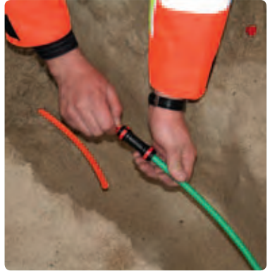
6. Fit the connector to the end of the duct that is to be used. Remember to mark the insertion depth on the end of the duct.
