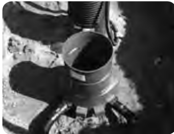
From the phosphorous trap, water is channelled to the distribution chamber, from where it is distributed to the land filter trench/infiltration system.
