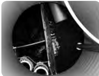
The chemical is dosed in the first sludge separator chamber.
