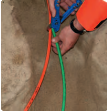
5. Adjust the length on each Opto Net duct to the length of the end of the duct that is to be used.
