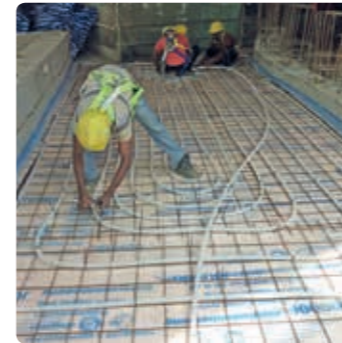
Radiant floor cooling for the conservatories: first developed in a thermal simulation, then transferred into practice
