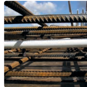
Pe-PEX pipes are integrated into the building structure
