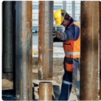
Ruukki steel piles are driven 28-30 metres into the ground. These serve both as the load-bearing structures to support the foundations and collect ground-source heat to heat and cool the building
