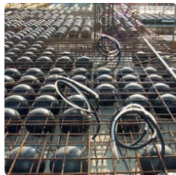
The Uponor TABS cooling system is incorporated into a BubbleDeck® construction
