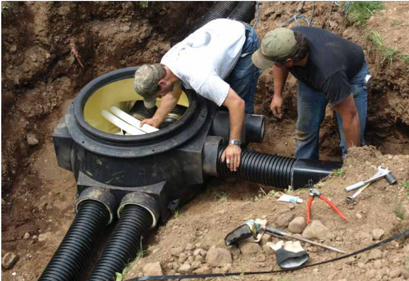
Figure 5-8: Ecoflex connection vault
