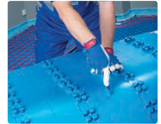
Additional panels for doorways and distribution areas
