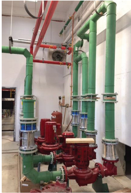
Figure 1-5: PP-RCT mechanical-room piping
