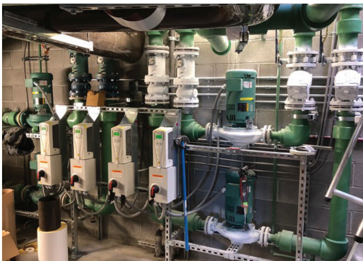
Figure 1-3: PP-RCT mechanical-room piping
