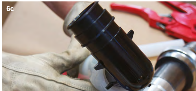
Insert ProPEX fitting into 2" Uponor PEX piping.
