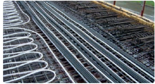
The Uponor Contec modules are installed in the centre of the floor
