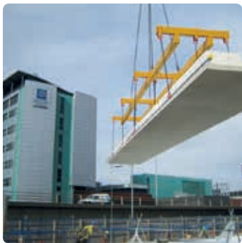
13,500 m 2 of Uponor TABS cooling in semi-precast concrete planks
